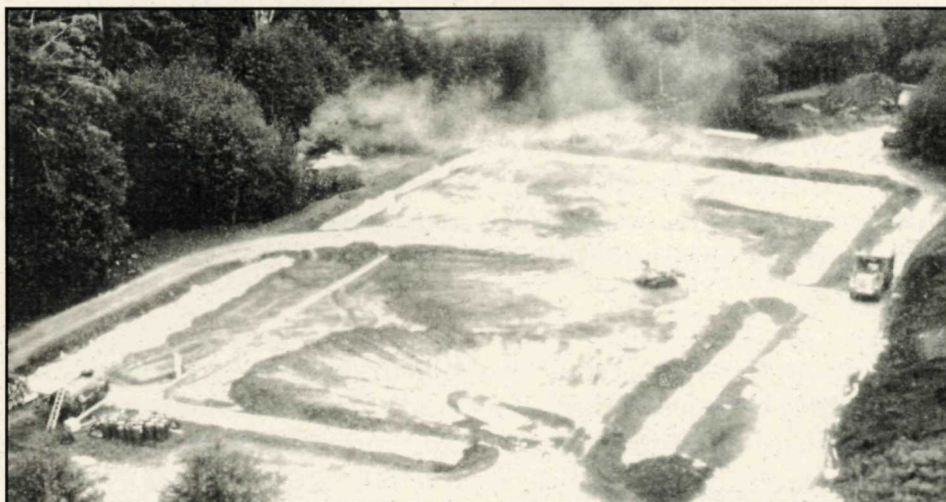
Constructing the 40m x 80m x 3m cell to hold impacted soils from various sites
