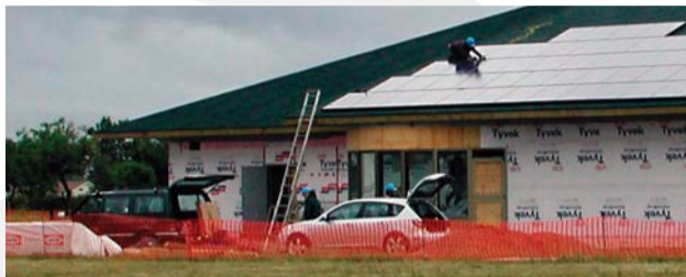
Photovoltaic cells being installed on the new visitor reception centre at Fort Battleford NHSC.
