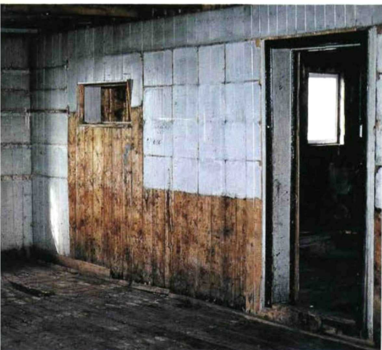
Shelf marks on an interior wall surround an opening that may have been a trading wicket. The floor is rotting away here, and in other parts of the lower storey.
