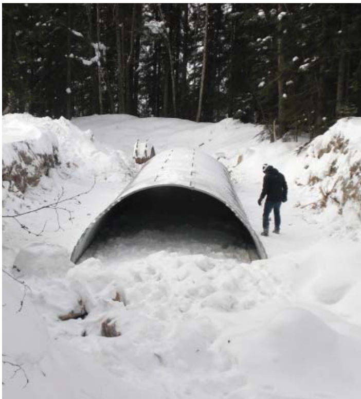
New arch culvert being installed on frozen Monarch Creek to restore aquatic connectivity (© Parks Canada / D. McNamara)
