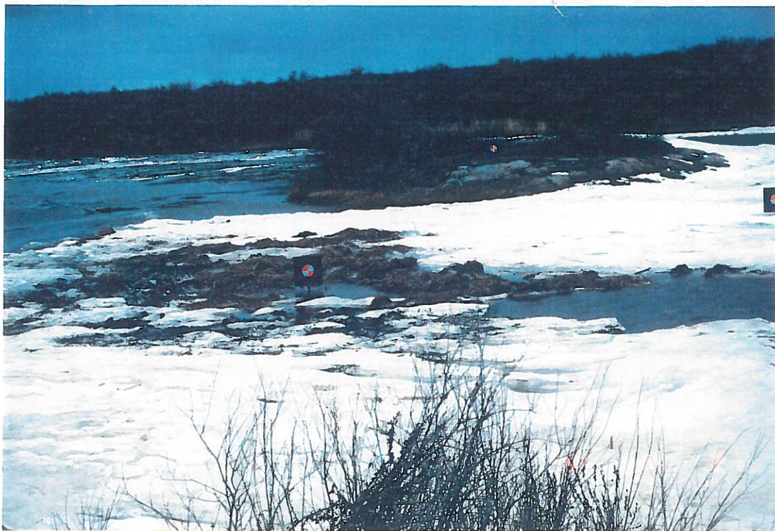
Photo 8: The south dam eroded away from the bottom up, with a channel finally developing through it's centre.
