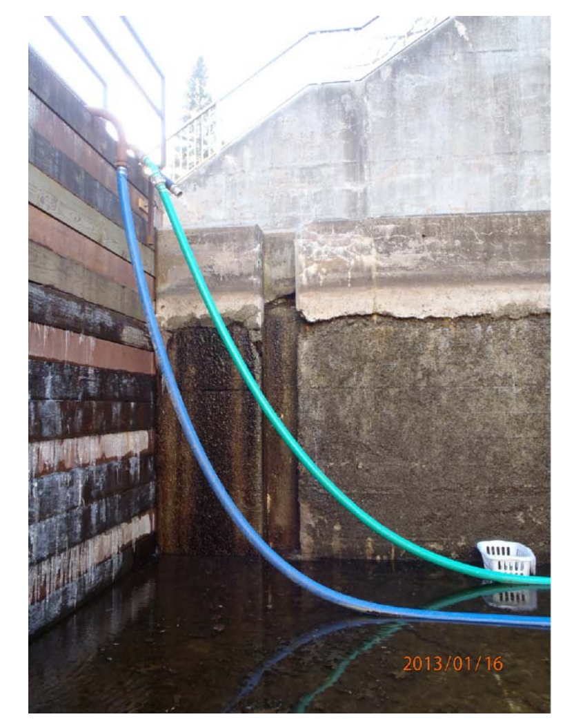
PHOTO SHOWS SERVICE STOP LOGS DEPLOYED IN OUTER GAINS AT LOWER GATES FOR DEWATERING SYSTEM
