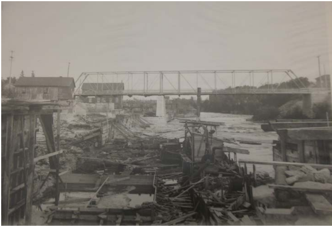
Appendix F: Construction of the dam, removing the wooden timber cribs and replacing them. Lakefield Historical Society: Delladone collection.
