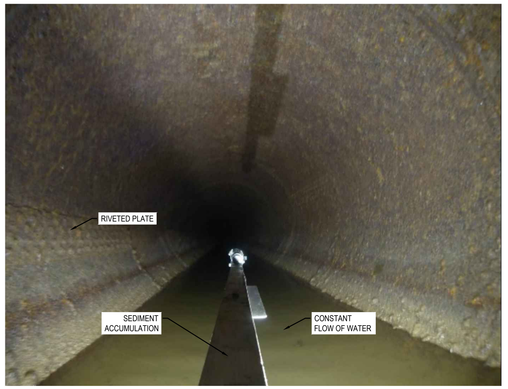
CURRENT PENSTOCK PIPE CONDITIONS SCALE: NTS
