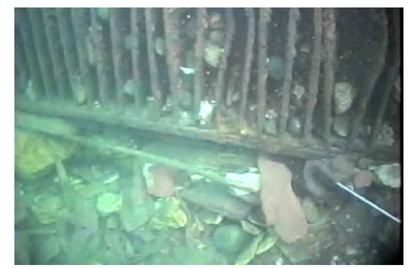
MISSING EXISTING BOTTOM STONE SCALE: NTS
