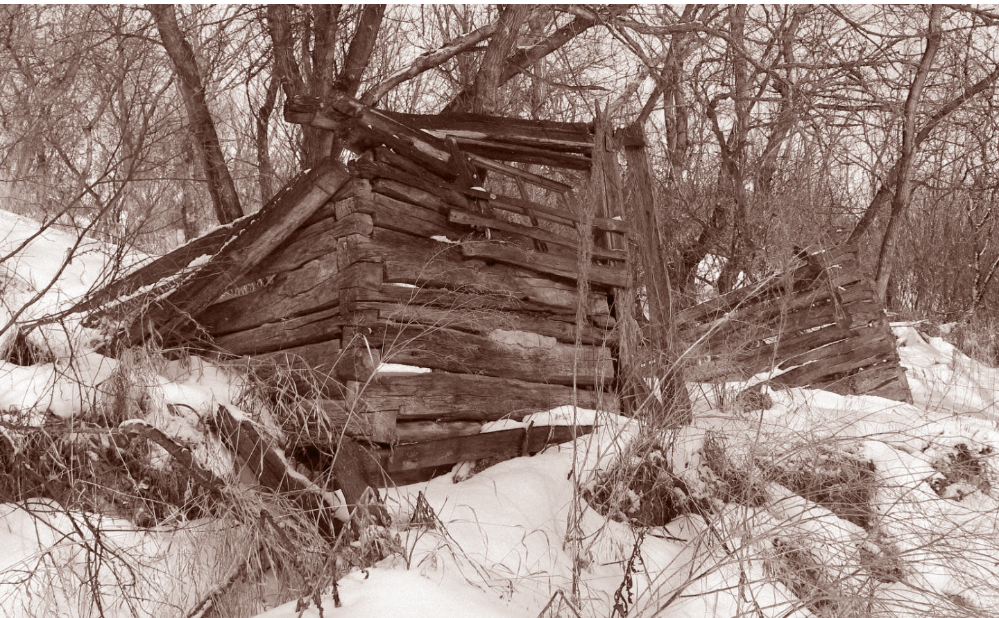
South side of the Doukhobor Dugout House in winter, 2006. Government of Saskatchewan, Bernard Flaman
