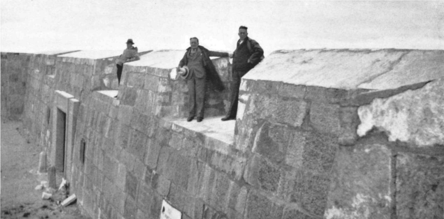
The fort in course of rebuilding by the Dominion Government. H. E. Cooper and W. E. Brown of the H B C stand in one of the embrasures. Beyond is the fort gate.
