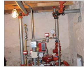
FIRE SUPPRESSION, STONE HOUSE BASEMENT PARKS CANADA / C. ARCHER / 2009
