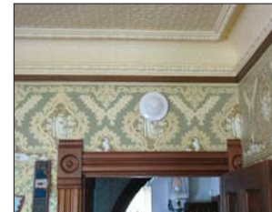
HEAT DETECTOR, STONE HOUSE PARKS CANADA / C. ARCHER / 2009
