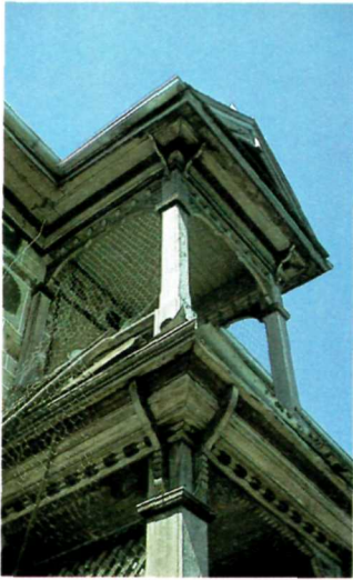
The balcony over the front entrance overlooked miles of prairie land. (Before restoration). Le balcon au-dessus de l'entrée principale dominait la vaste prairie (avant la restauration).
