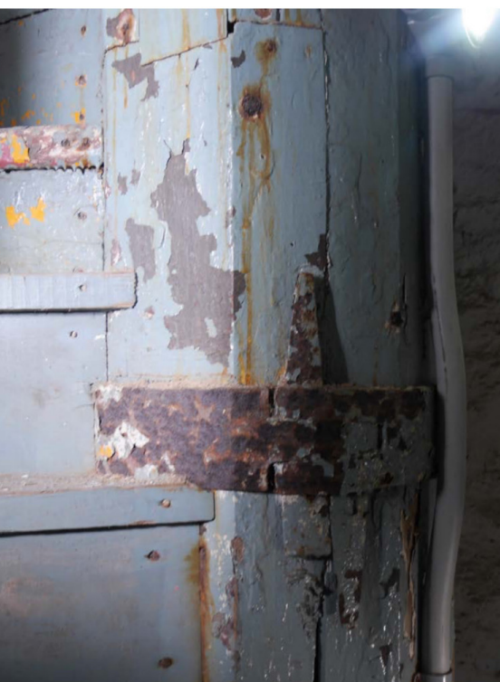
When THA Architects and RJC Engineers arrived, the interior of Sambro Lighthouse had been badly deteriorated by the elements. | Avant l'intervention de THA Architects et de RJC Engineers, l'intérieur du phare Sambro avait été gravement endommagé par les éléments.
