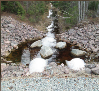
Ponds built at every culvert for fish and amphibians.
