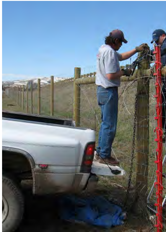
Figure 31: Wildlife fence along Interstate 90 near Bozeman, Montana (© Marcel Huijser).
