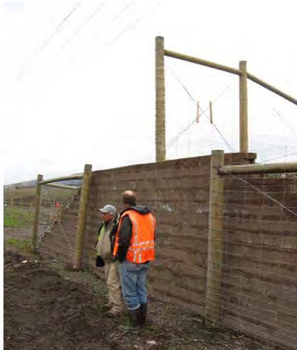
Figure 43: A jump-out along a 2.4 m (8 ft) high fence along U.S. Highway 93 in Montana (© Marcel Huijser).
