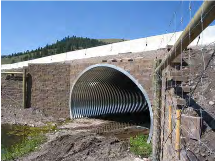
Figure 54: Wildlife underpass along U.S. Highway 93 on the Flathead Indian Reservation, Montana (© Marcel Huijser).
