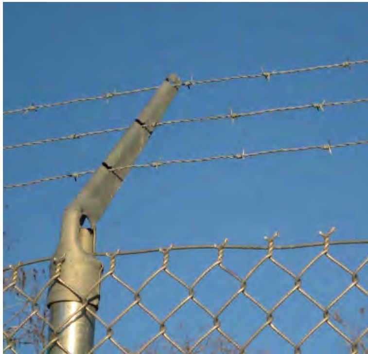
Figure 34: A 3.4 m high chain link fence along SR 29 in southern Florida was equipped with three strands of outriggered barbed wire to prevent Florida panthers from climbing the fence (© Marcel Huijser).
