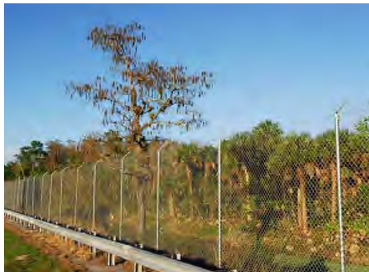
Figure 33: A 3.4 m high chain link fence along SR 29 in southern Florida designed to prevent Florida panthers from entering the roadway and to guide them toward underpasses (© Marcel Huijser).
