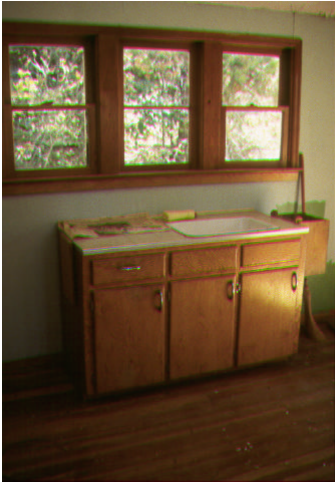
Figure 5 Interior view of the kitchen area, Mount Daer Fire Lookout, Kootenay National Park (1473T-5t).
