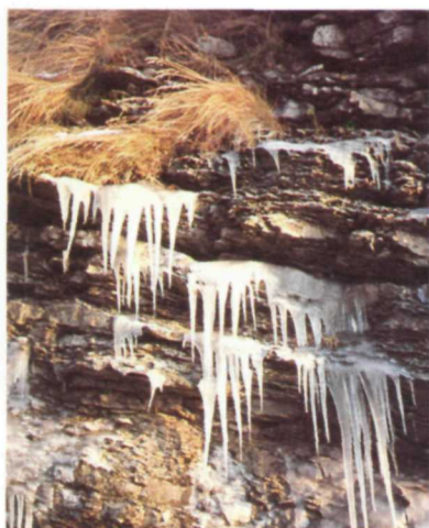
Water seeping between rock strata
