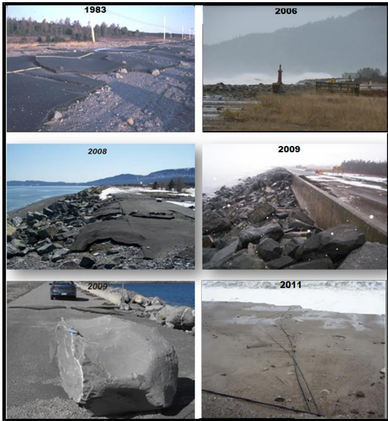
Figure 2. Typical damage observed over the years on Route du Banc and related infrastructure – Source: Parks Canada.
