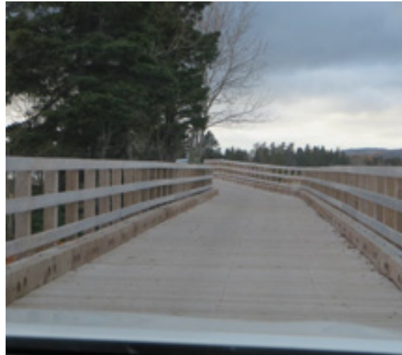
The new footbridge/road in La Penouille, constructed on piles to withstand flooding
