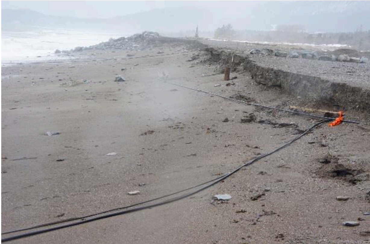
La Penouille, 2011: Storm damage to pavement and underground power lines
