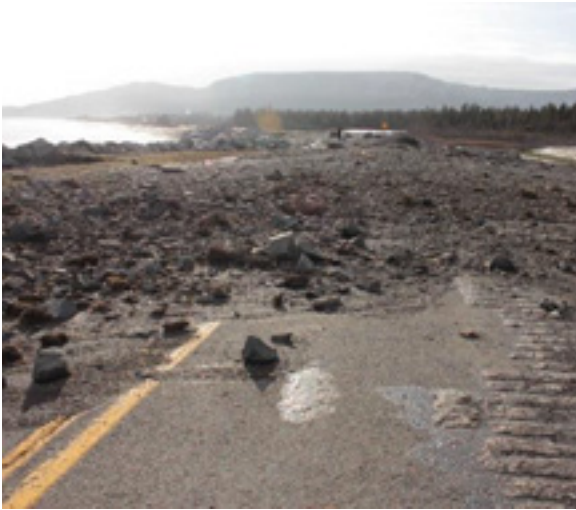
In Penouille, two storms in one week destroyed the road in 2010
