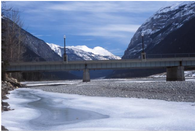
Bridge over Kicking Horse River into Field Townsite. Photo: Parks Canada, S.Morris 2005
