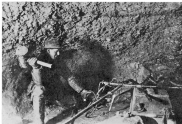
The photograph (showing pipes) was taken 88 feet below the surface.
